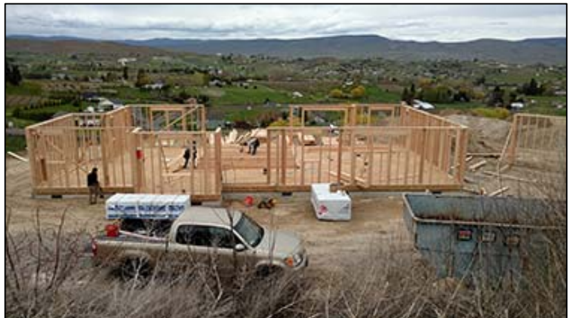
Photo from Copper Hills Construction [enlarge] Rural developments, like this home under construction in Selah, often rely on permit-exempt wells for drinking water.
